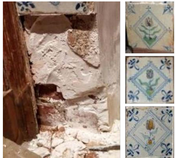
Figure 15: (Left) After de-installing tiles, it was revealed that a thick layer of plaster attached the tiles to brick, and that water damage and salt migration stained tiles like 1969.4722.002 (top right), caused structural cracks like those on 1969.4722.027 (right center), and spalling glaze like on tile 1969.4722.031 (bottom right).
